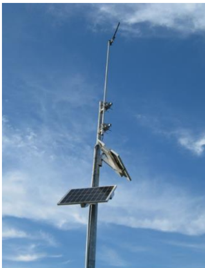
Figure 4: Portable flow monitoring station solar panels and directional antenna
